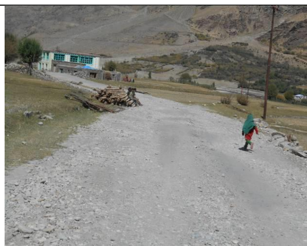
BT washed away at Km 60+800
